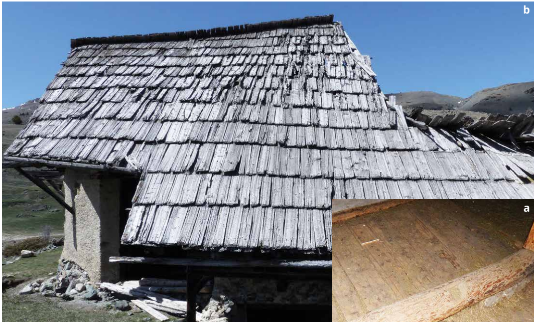
↑ Figure 5. a) A roof board has been reused in an interior floor (the white scale on the board measures 20 cm). b) This farm is located at an altitude of 1390 m. These alpine roof boards are very recognisable because they have two gutters on each long side to facilitate snow drainage (Photo by L. Shindo; image modified).
