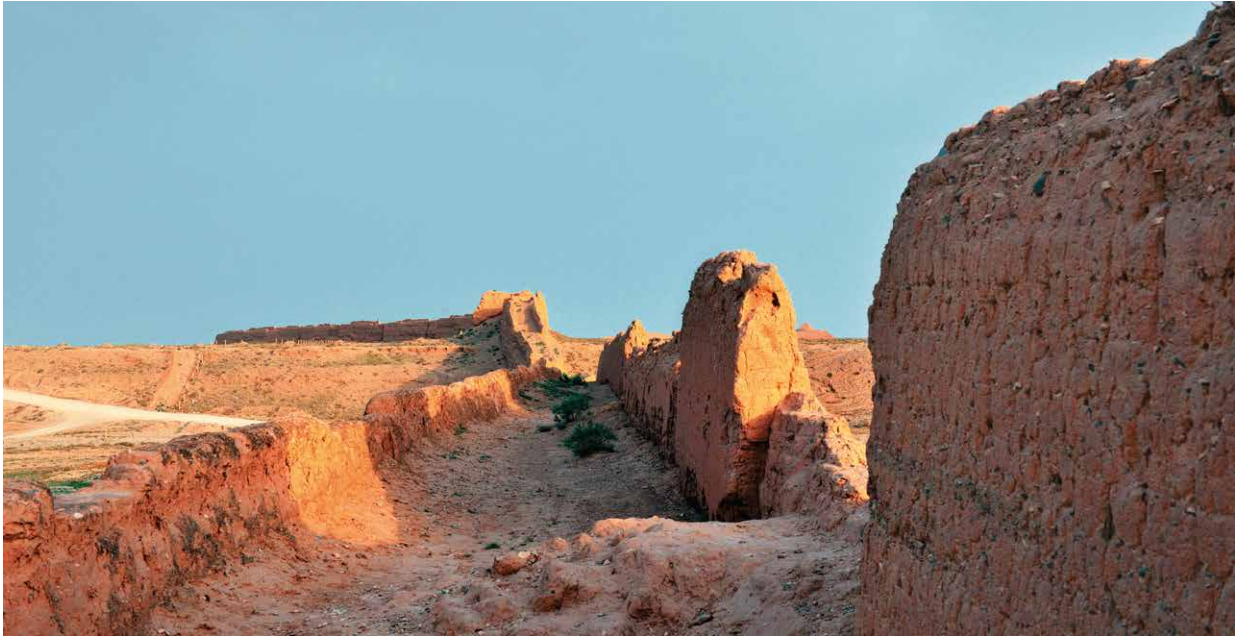
Figure 3. In western province like Ningxia the Ming Great Wall was built of rammed-earth and has already deteriorated considerably (© Wang Yungang).
