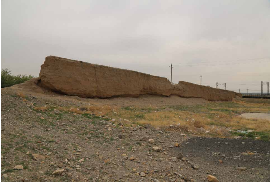
Figure 2. The wall eroded, the Old North Wall.
