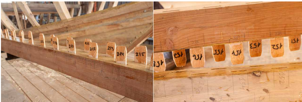
Figure 4. Detail of the third starboard wale showing corresponding numbers of the mortise-and-tenon joints (Photo A. Efremov).
