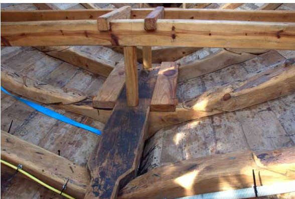
Figure 10. The reconstructed mast step assembly during construction. Pipes of the bilge pump are seen in the foreground (Photo J. Tresman).
