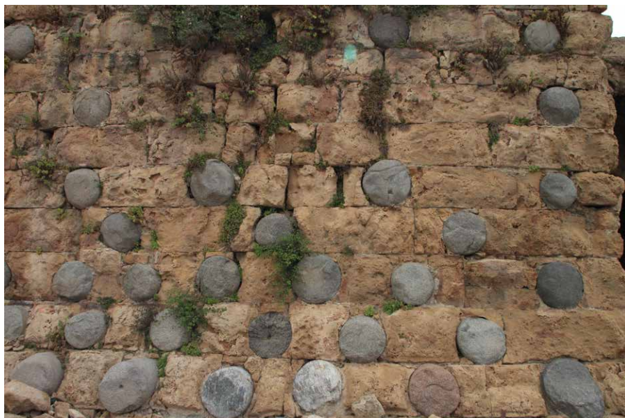
Figure 9. Columns embedded in the walls of the sea castle of Sidon (Photo P. Antaki-Masson).
