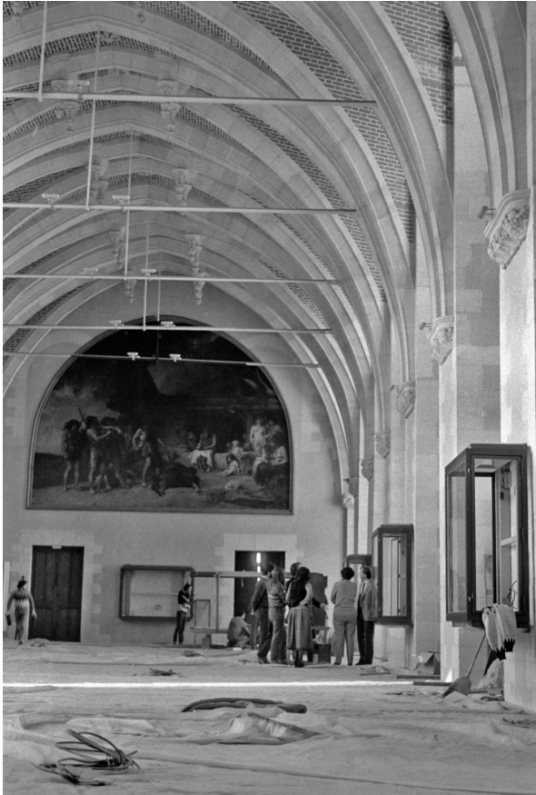
Fig. 3 Restoration works in the Comparative Hall, around 1980-1982 (MAN, Service des ressources documentaires).
