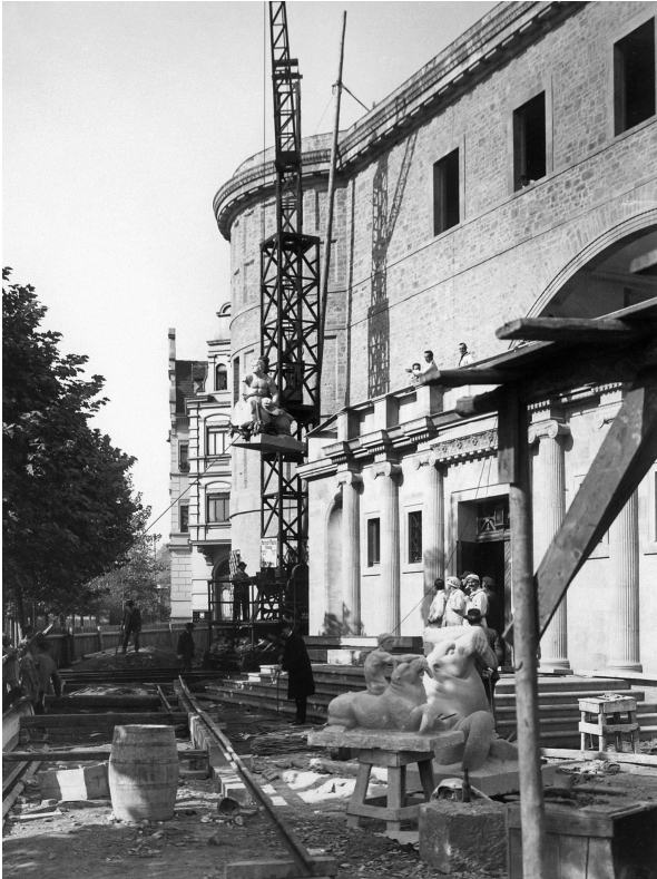
Fig. 2 Building site of the Museum (1913). Germany's first purpose-built Museum of Prehistory opened on 9 th of October 1918, about a month before the armistice (© LDA).
