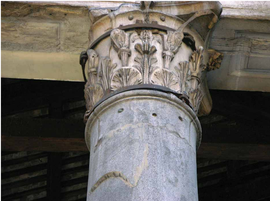
Figure 3. Pantheon, Rome. Detail of one of the porch columns of Mons Claudius granite with rippled joint (Photograph: the author).
