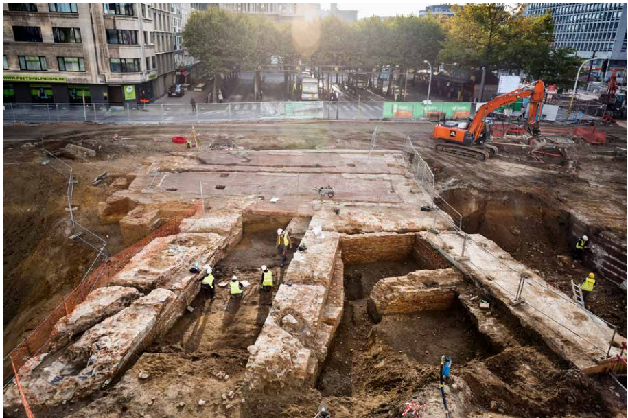
Figure 4. View from the west of the excavation of the nineteenth-century casemate, with artillery floor and postern in place (Lucid).
