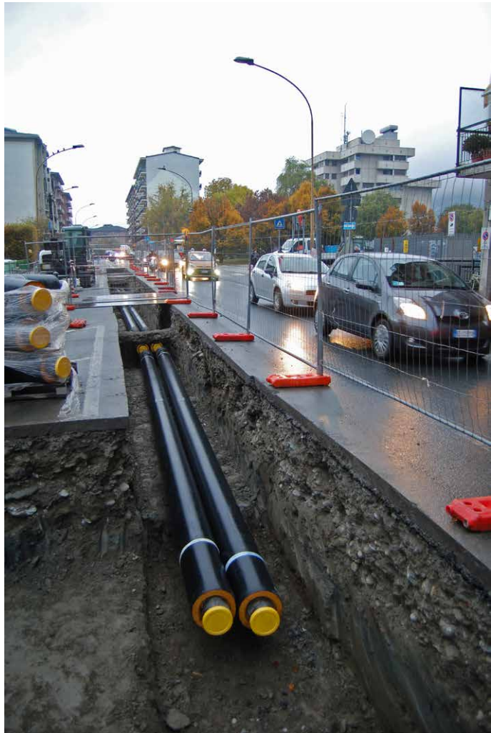
Figure 7. Telcha. An example of the installation of the rigid tubes of the Telcha project in Aosta (Akhet srl).
