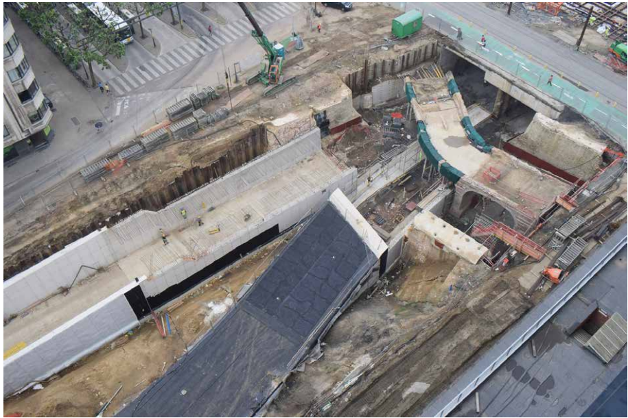
Figure 10. Aerial picture of the construction of the tunnels below the vaults of the bridge (City of Antwerp, archaeological department).
